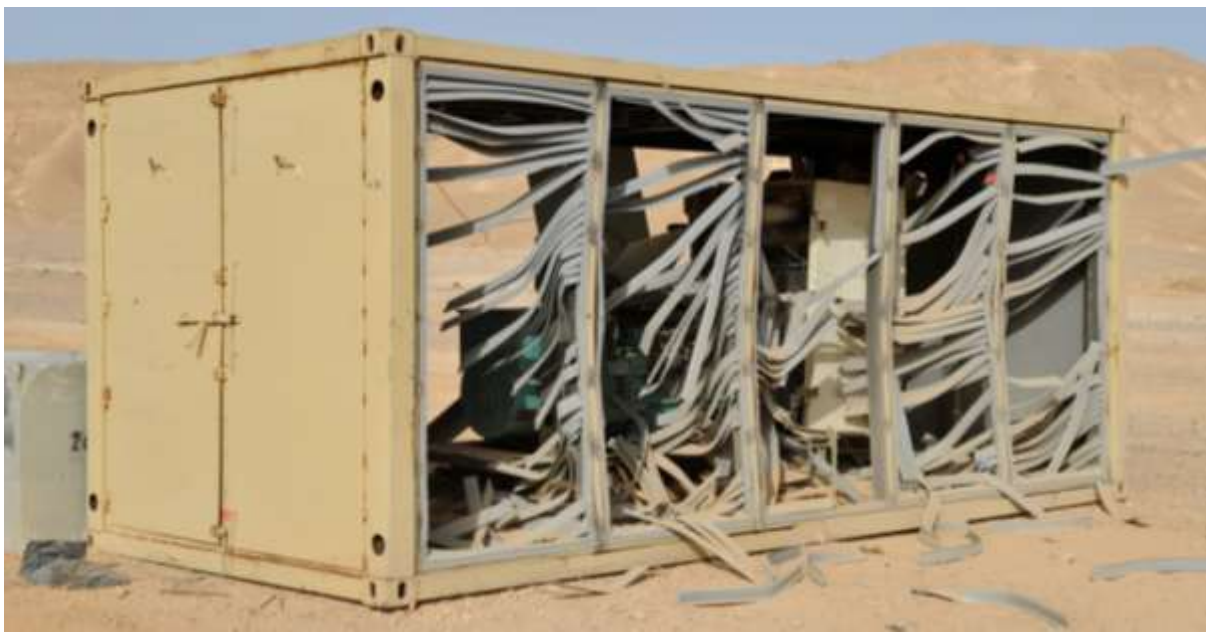
Figure 33 Generator and enclosure after test
