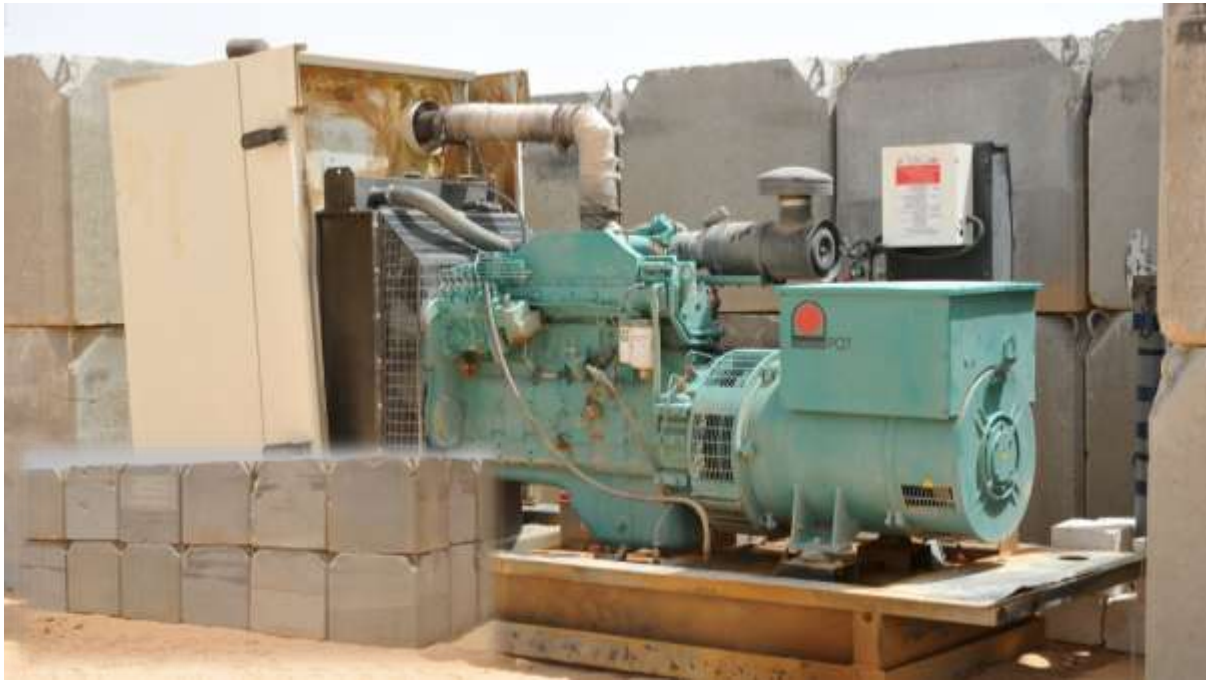
Figure 46 Generator before test
