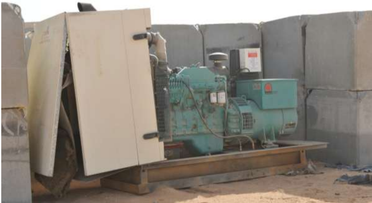
Figure 41 Generator after test
